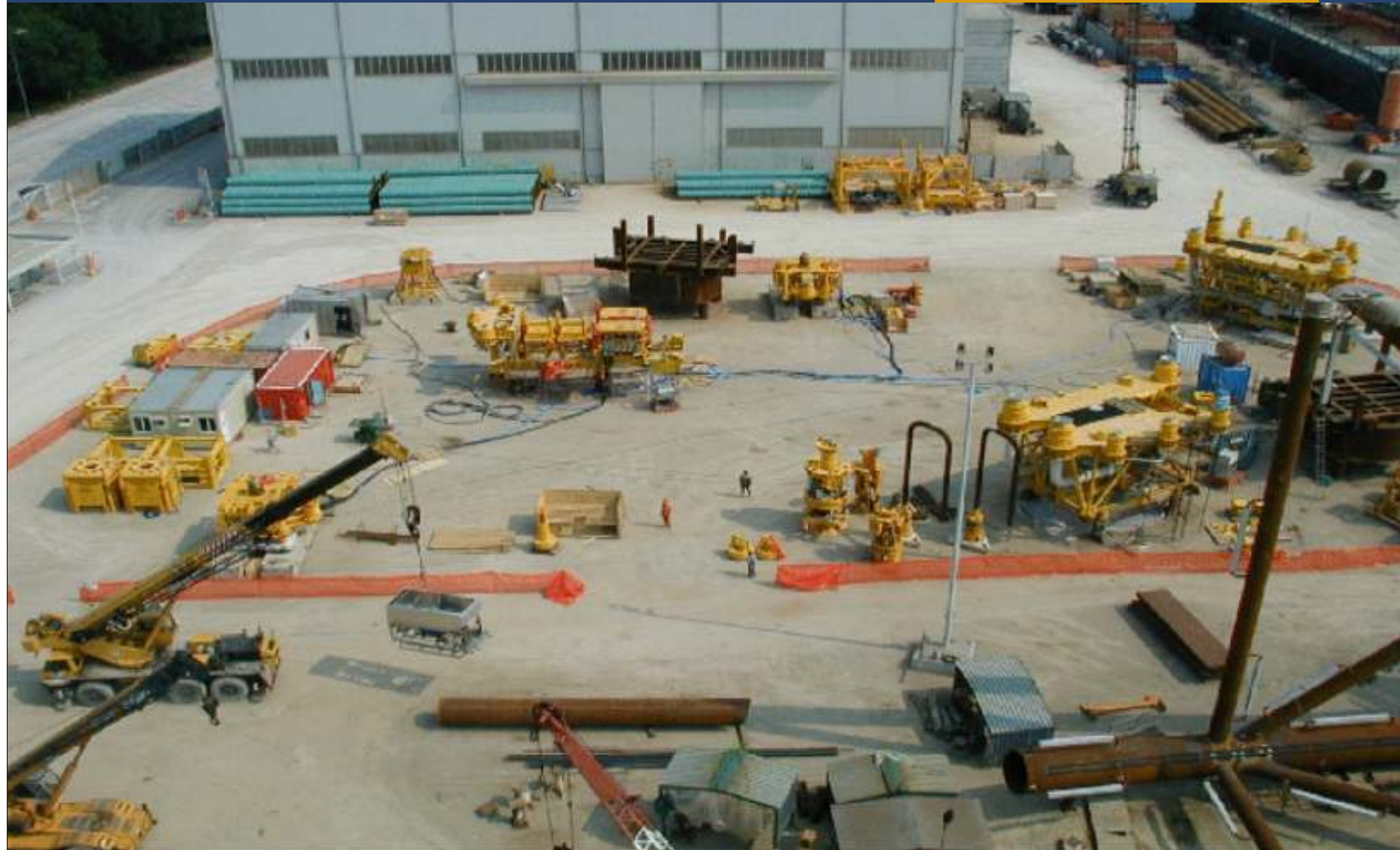
The Reliance KG D6 Deepwater Gas Field Development Project involved the installation of 125,000 metric tons of sub-sea equipment, deployment of over 80 offshore vessels, 20,000 people at the peak of the project, more than 200 consultants and service providers, and over 50 million person hours.
